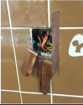
< Covers missing from socket sin Pool/Wet change side
